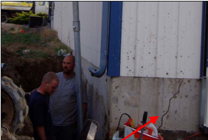
4 inches of settlement caused the foundation wall to crack.
