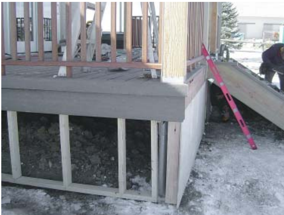
Figure 5. To make the room addition better match the existing house and its concrete foundation, the author uses a skirting system made from pressure-treated lumber covered with cement board. Seams and screw holes are skim-coated with mortar to give it a monolithic appearance.
